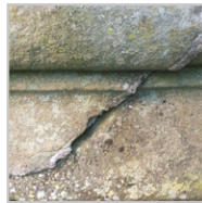
Cracks in Stone
